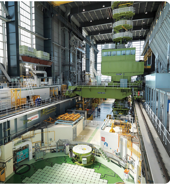
Above image: Pile cap and fueling machine, Hunterston B. Image supplied courtesy of EDF Energy.
